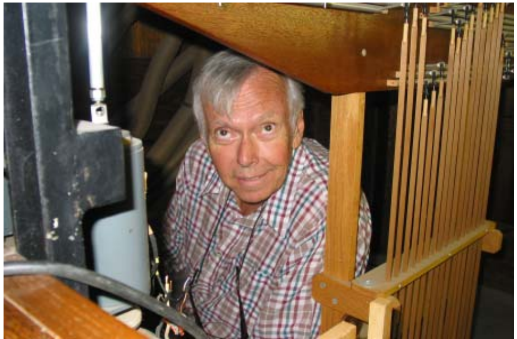
(Above) Ross Doddington tucked into the tiny space behind the Organ Pipes to maintain the instrument and replace some capacitors that had lost their capacity for being capacitors.
